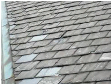
A close-up photo of our roof showing deteriorating and missing slates
